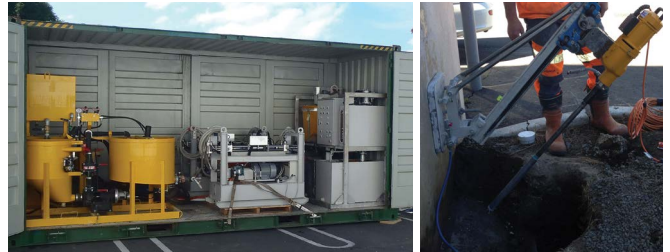
Above, left: Typical JOG site control centre with computer controls, slurry tanks and pumping equipment. Above, right: Angular insertion of JOG injector.
